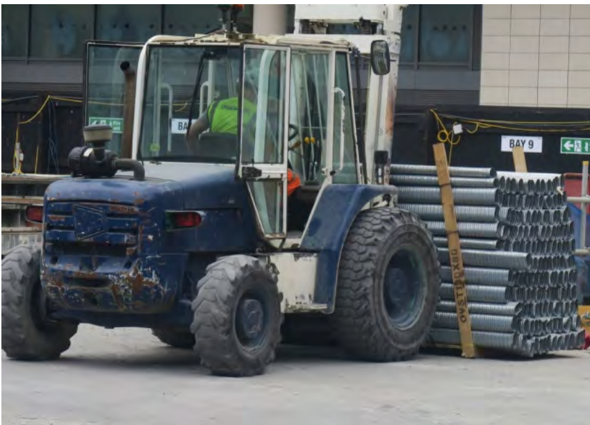
Construction staging work being carried out at Cuba Street without planning permission, says council. Picture: Mike Brooke
